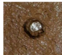
The cone had remained in the hole for inserting a metallic expansion anchor and its cone.
