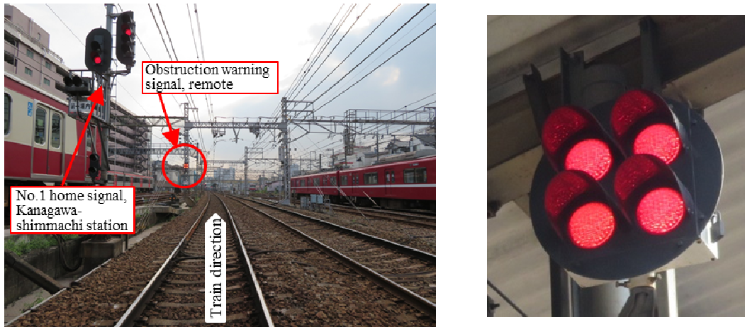
Figure 5. Installed status of the remote OWS, left, and display in the middle OWS, right.
