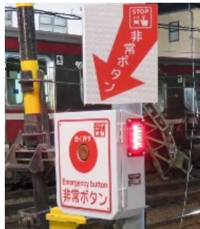
Figure 4. The operating device, i.e. , the push button, of the Level crossing
