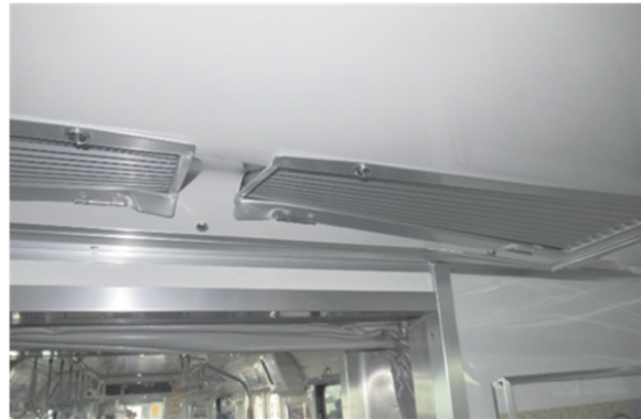
Distortion of the ceiling panels in Shin-Sugita station side of the 4th vehicle
