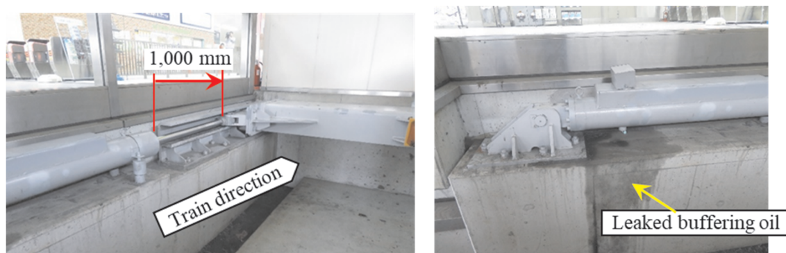
Figure 3. Status of the hydraulic buffering device after this accident
