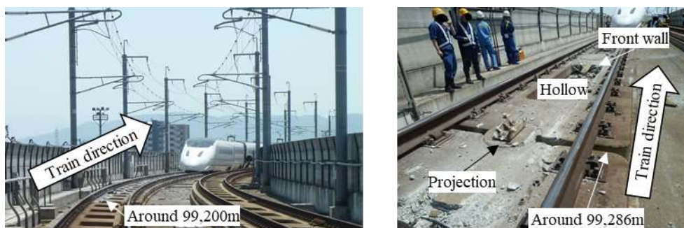
Figure 5. Damaged status of frame shaped slab.
