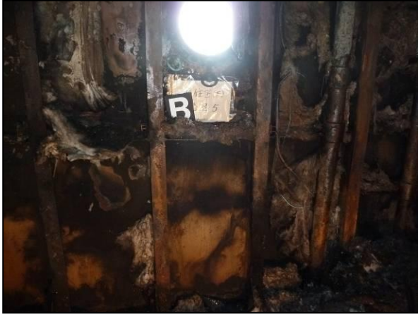
Photo ⑪ "Forward Port side cabin: Severely Burned"
