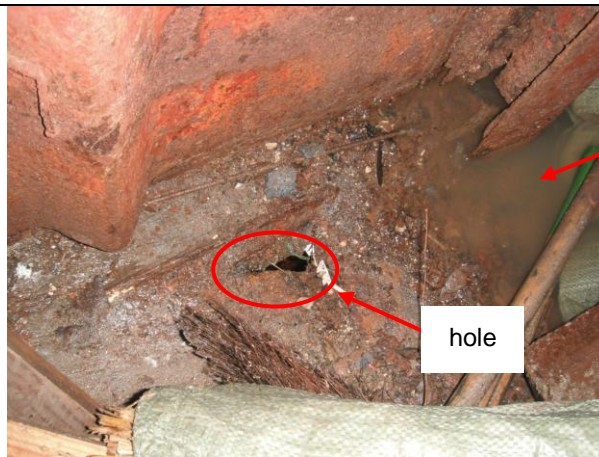
Photo 9. Hole on the bottom of store room
