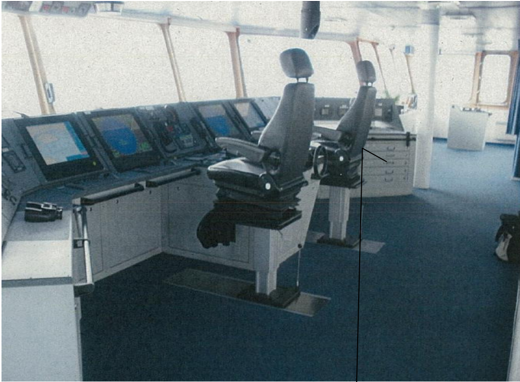
Photo 1: Appearance of the Wheelhouse (around the Chair)
