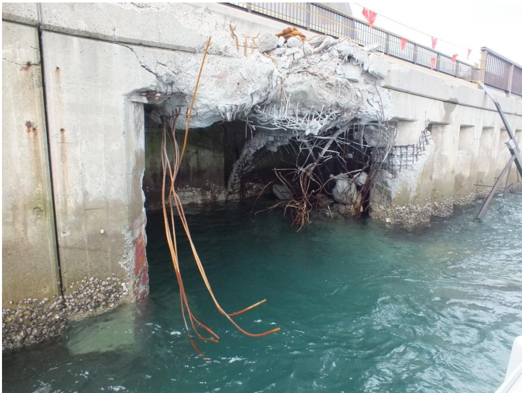
Photo 4: Damaged Part of the Sea Wall
