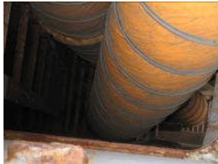
“spiral ducts in hatch entrance”
