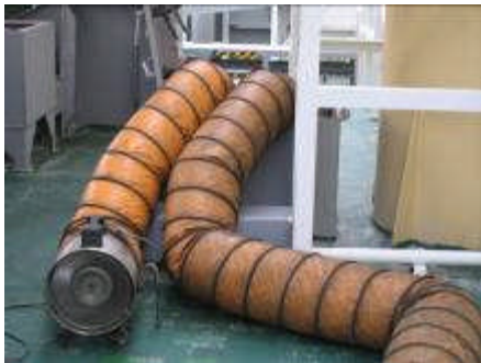
“forced draft by forced draft fans and spiral ducts”
