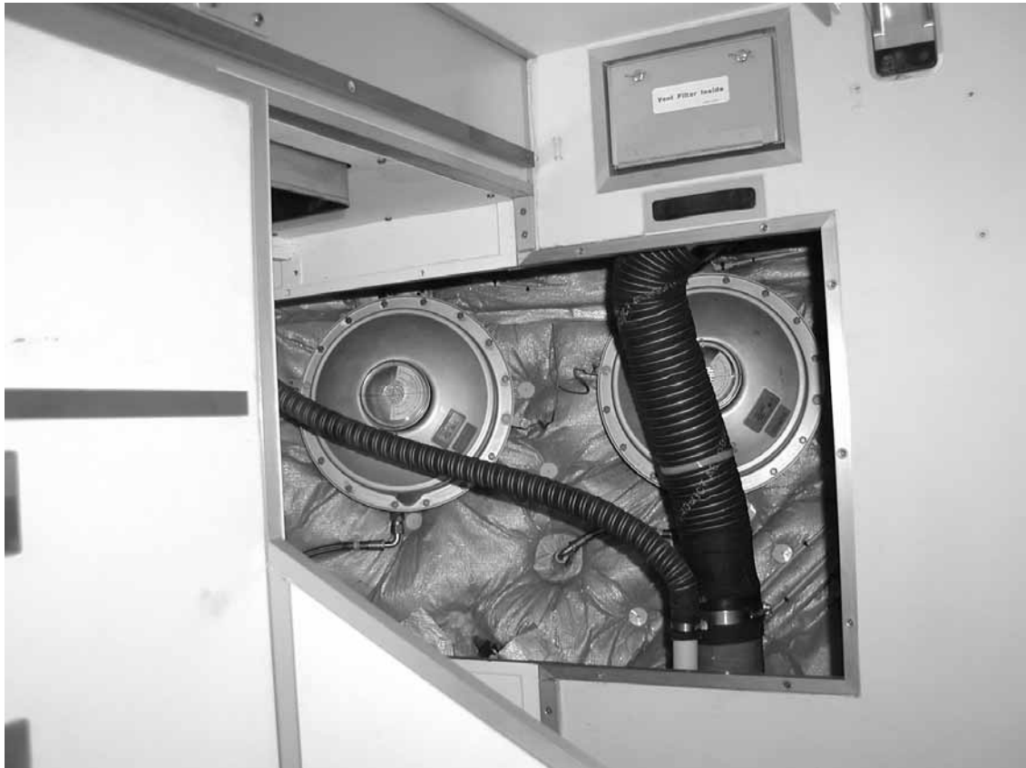
Photograph 1 Safety Valves front side
