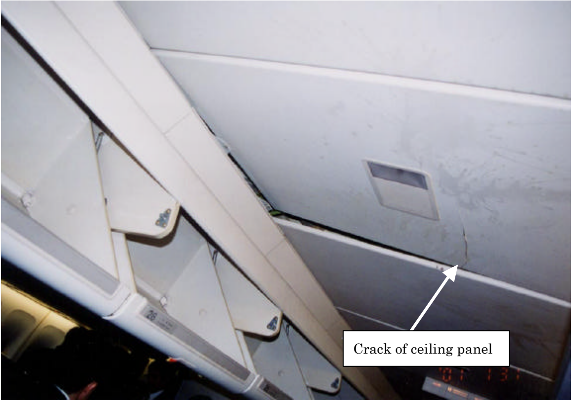
The damage of ceiling panel over right side pass way seat No. 26(view from backward)
