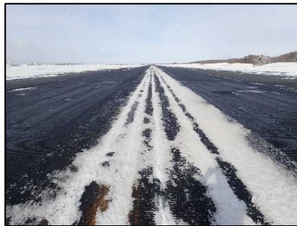
Photo 2 - Condition of South-side runway (Pictured at the time of assessment after the occurrence of the serious incident)
