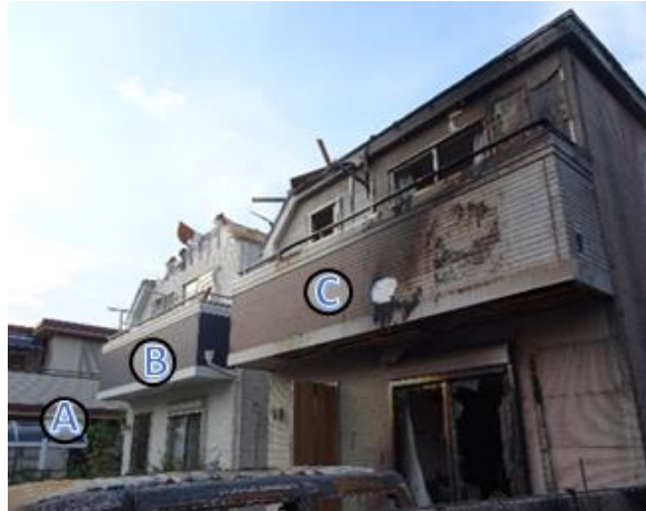
Photo 2.4.2-4 Fire Damage of House C
