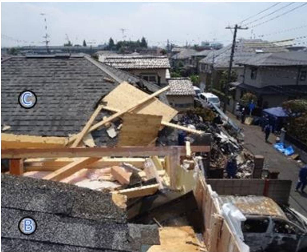
Photo 2.4.2-3 Damaged Roof of House B and Roofing Materials Scattered on House C
