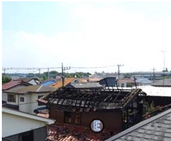
Photo 2.4.2-6 Fire Damage of House E
