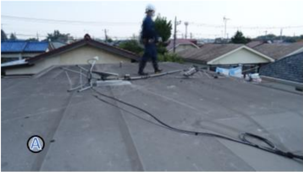
Photo 2.4.2-2 Collapsed TV Antenna of House A
