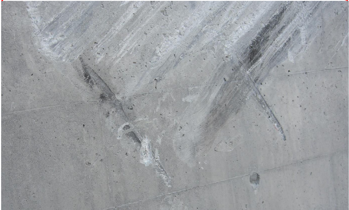
Photo 3: Propeller Slash Marks on Revetment Wall Surface
