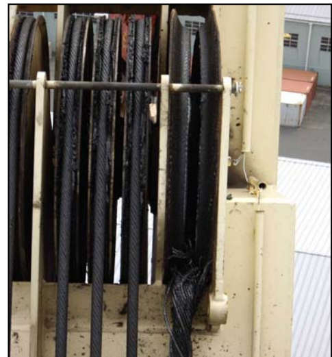
Sheaves at the end of Jib (Crane No. 3)
