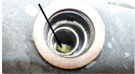
Side surface of valve base frame, that came off from the base hole, facing upward
