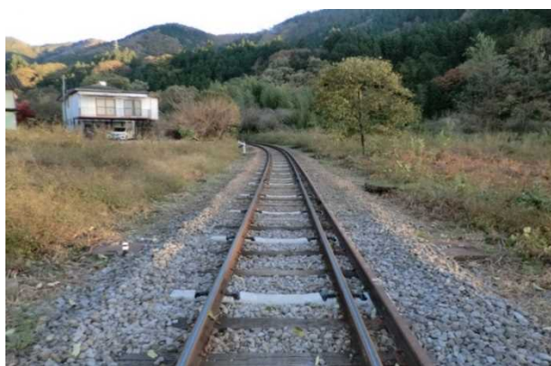
Figure 8: Example of partial replacement with PC sleepers
