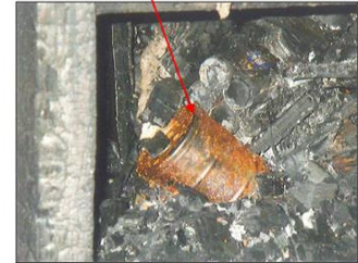
Ashtray Found under Stairway
